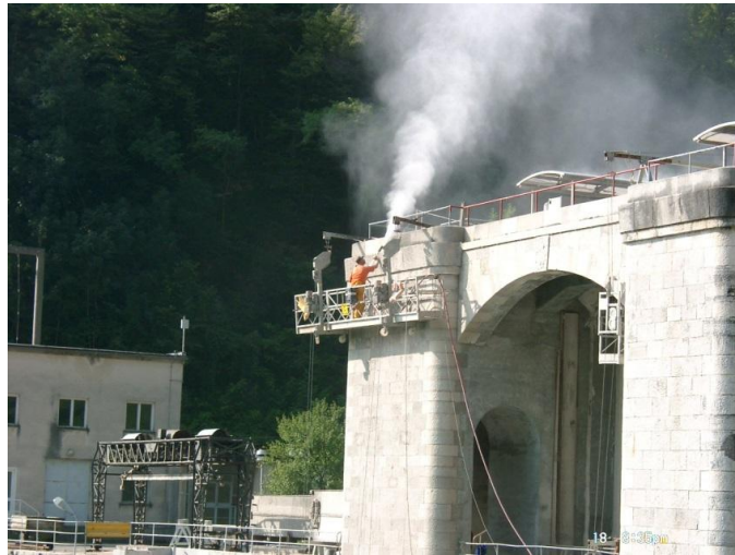
Figure 7 Sandblasting of stone facing on the right pier at the deck level (121m) in 2006
