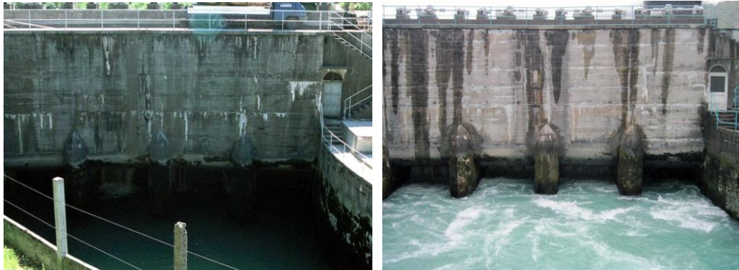
Figure 5 Intake structure HP Plave 1 before rehabilitation in 2004 and five years after it
