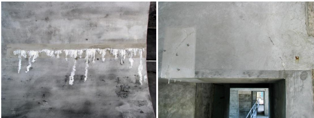
Figure 8 Reappearance of small number of cracks (in 2011)
